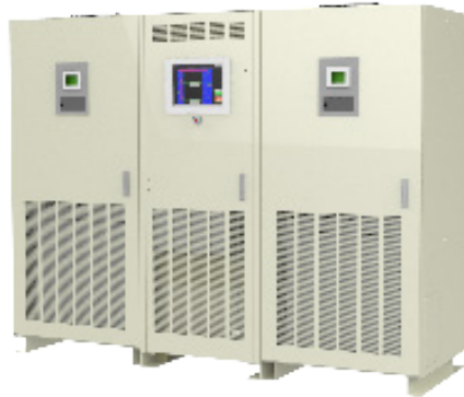
Paralleling Cabinet w/ UPS
