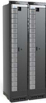
Available in High Power Density Configuration Combining Three Battery Strings in Two Racks
